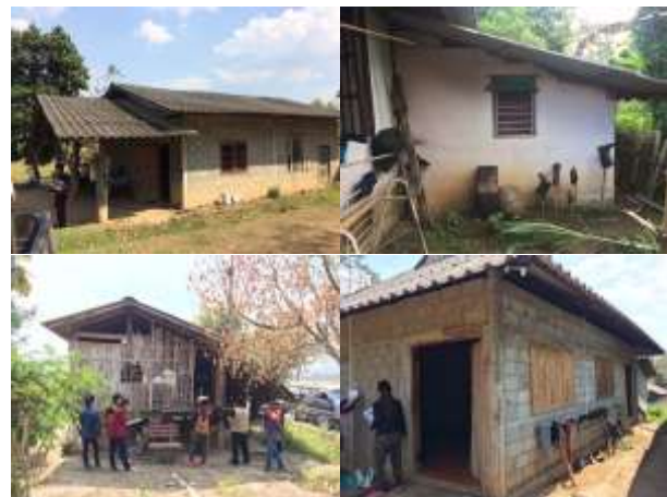
Fig 1. Surveying the damaged houses
